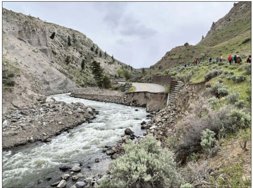
Field trip participants inspect the 2022 flood damage to Highway 89 connecting Gardiner, Montana, and Mammoth Hot Springs at the biannual Yellowstone Volcano Observatory meeting in May 2024. Yellowstone National Park is abandoning the old highway and evaluating a new route, hindered by park restrictions, physiographic barriers, and Yellowstone's potential to generate cascading hazards. The MBMG plans to map the massive landslide complex impacting the north entrance to the park as a fiscal year 2025 STATEMAP project.
