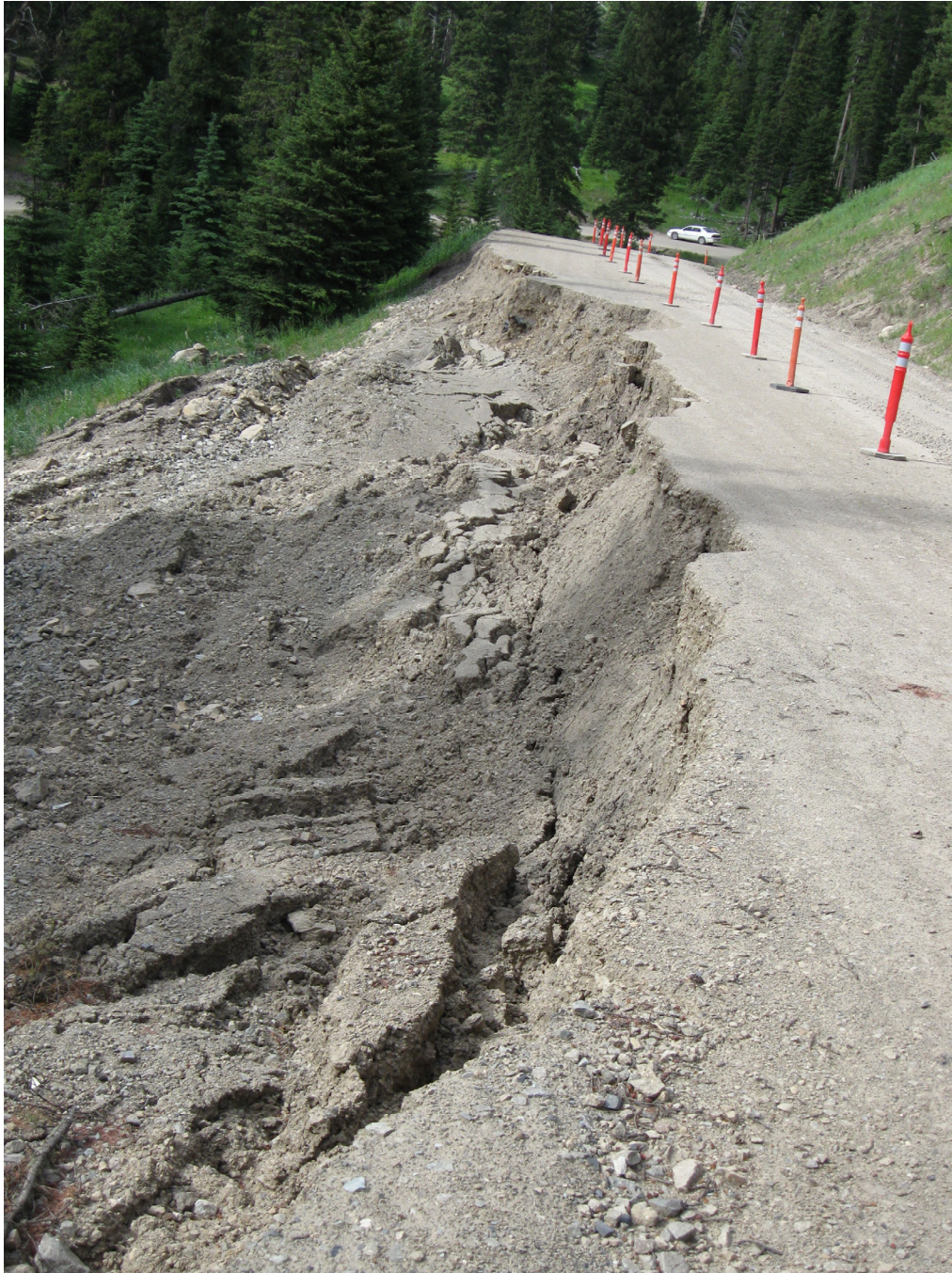
Figure 2. Landslide along Jack Creek Road in northwest part of map area (July 2008 photo).
